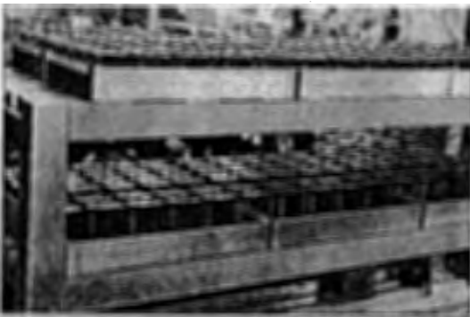
Fig. 5.64 Initial charging plant (Y. S. B.)
